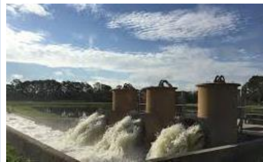
Storm water pumping stations
