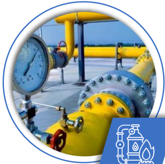
City Gas Distribution
