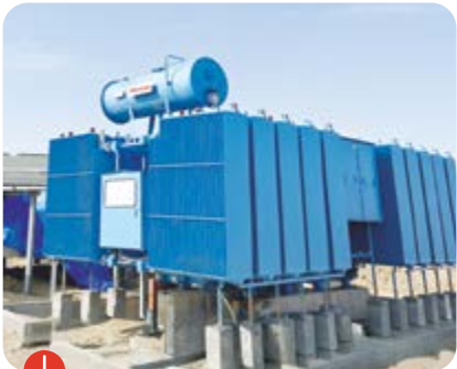
↓ Inverter Duty Transformers
