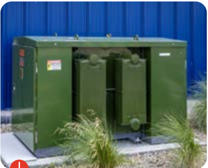
↓ Pad Mounted Transformers
