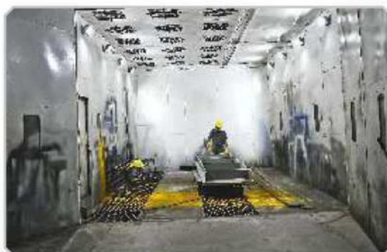
PAINT BOOTH UNIT
