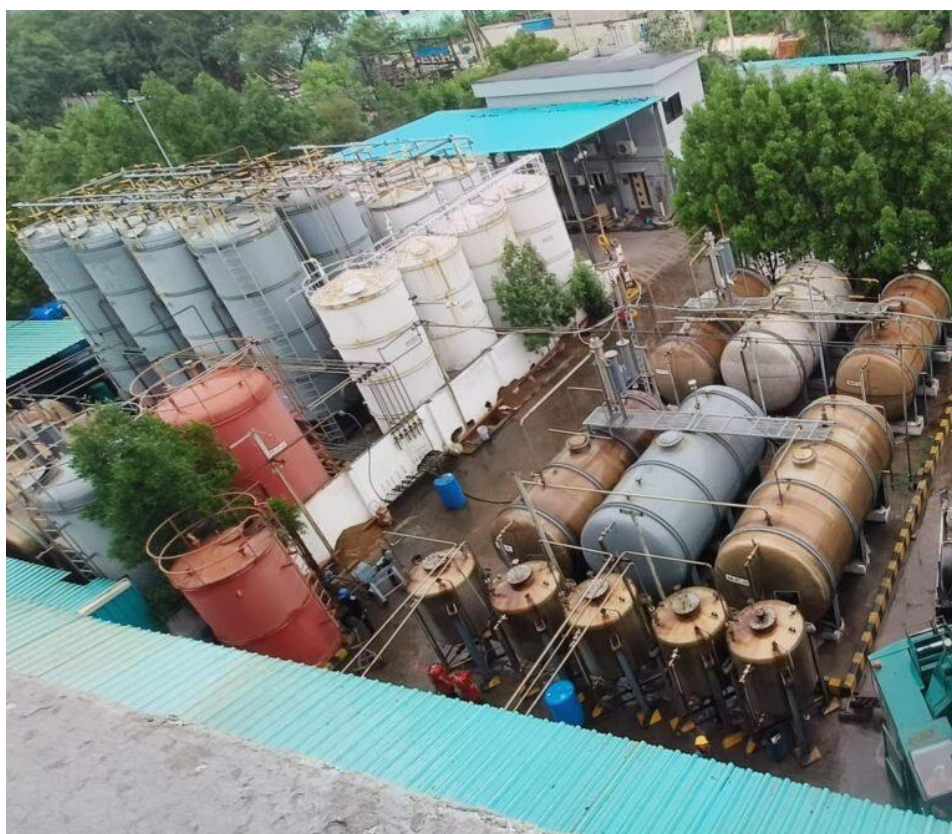
Storage tank farm holding recovered and traded solvents ahead of dispatch.
