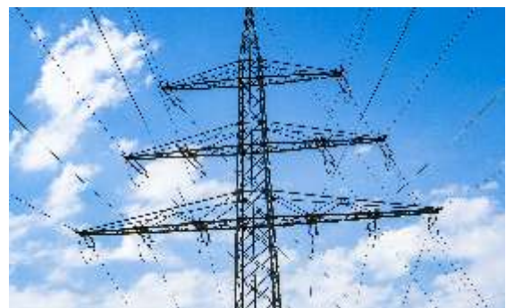
HV/EHV Operation Maintenance
