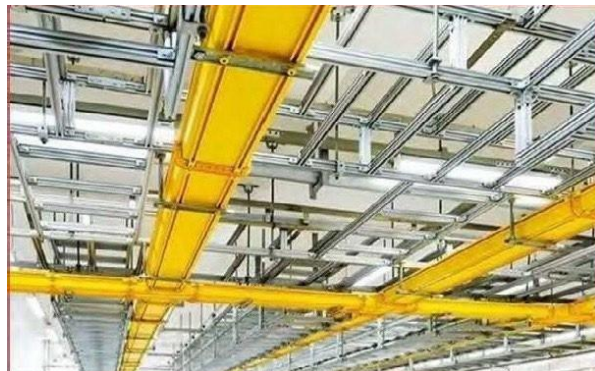
Wire forms and cable management
