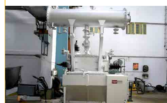
8MVA, 33/11kv Power Transformer
