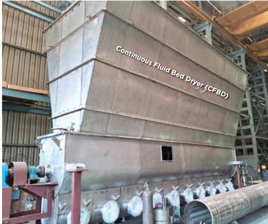
Continuous Fluid Bed Dryer (CFBD)
