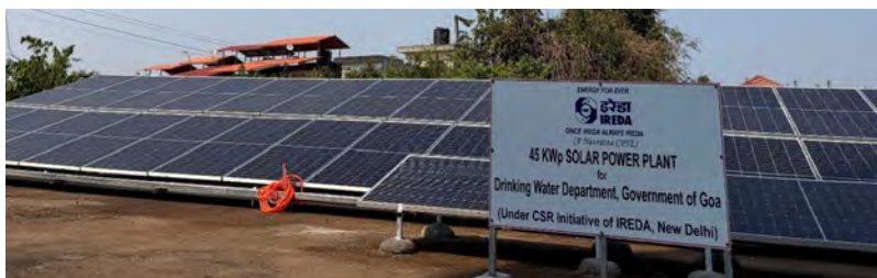
45 kW on-grid solar power system at a water pumping station, North Goa
